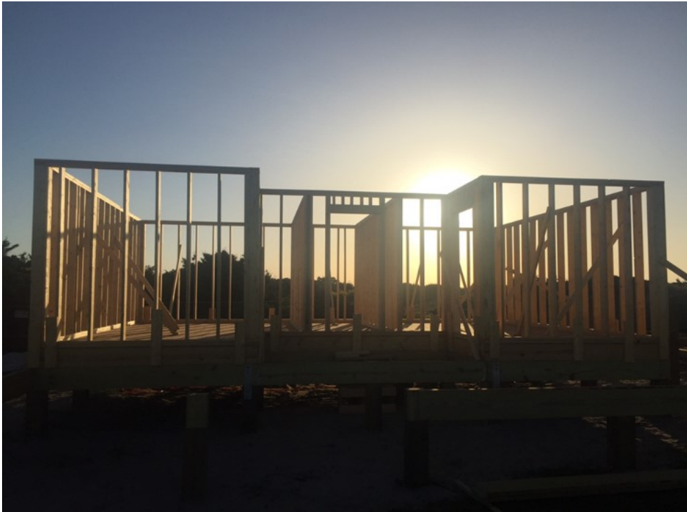
The restroom facility at the Ocracoke Beach Access is starting to take shape. The new facility is currently scheduled to open at the end of June. Portable restrooms are available on site.
